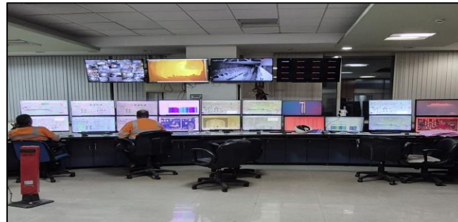
Central Control Room (CCR) The CCR is the plant's digital hub, continuously monitoring and optimizing all key processes
