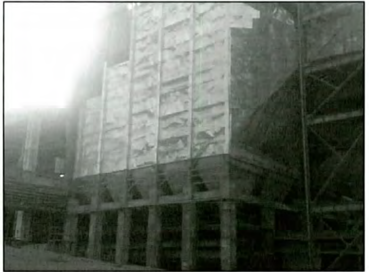
ESP at Cooler
