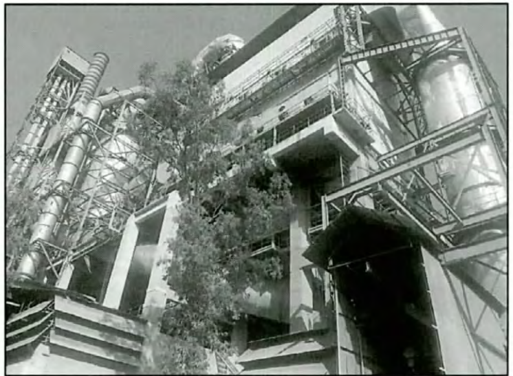
Hybrid Filter at Cement Mill
